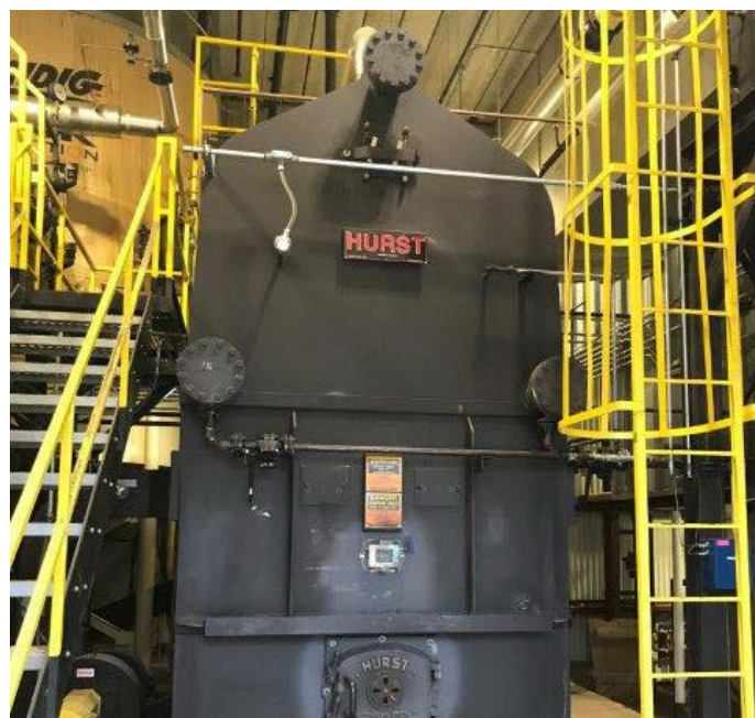
Cohasset (US) Wood Fired Steam Boiler
