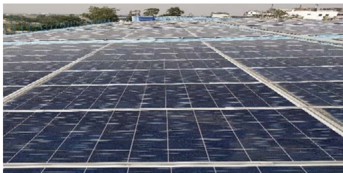
Haryana Onsite Energy Production
